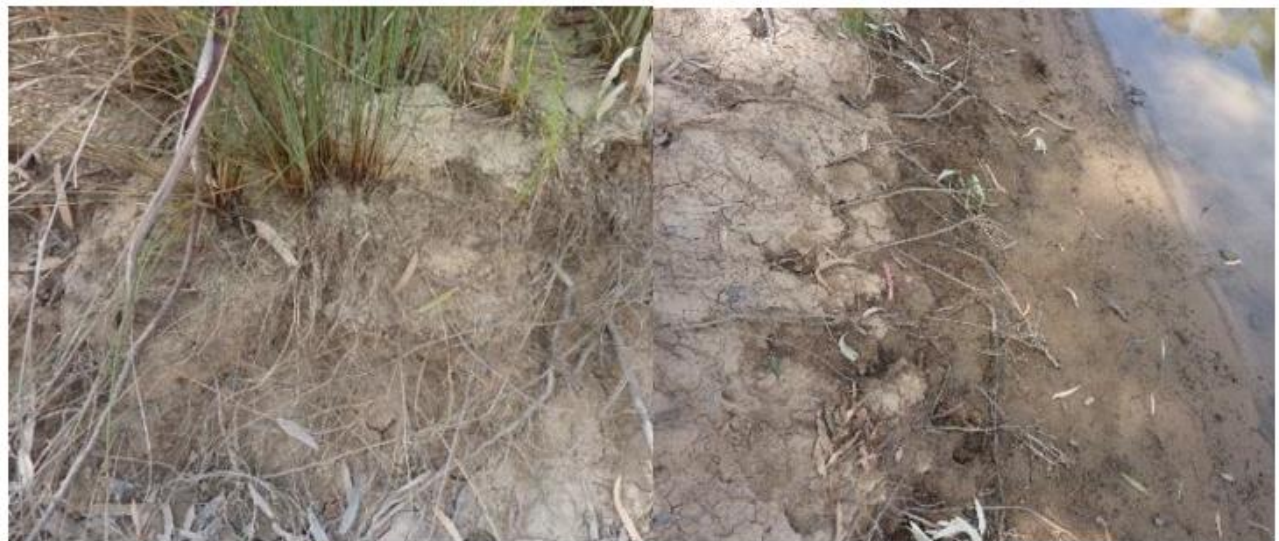
Figure 7-4 Signs of erosion along the lower bank.
