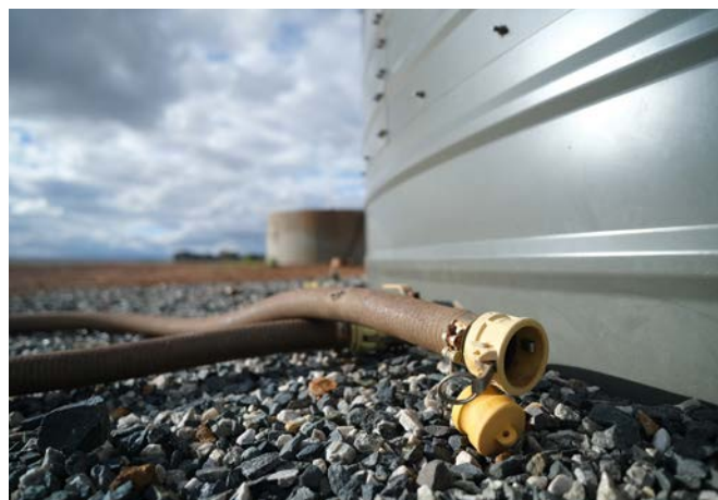
Image: Rainwater tank
