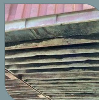
Soil on container underside
