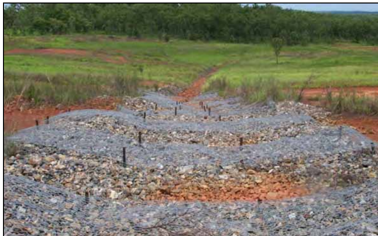
Figure 1 Longitudinal drain in the cap of Dyson's Open Cut. Significant signs of subsidence can be seen in the vicinity of the single tree located towards the mid-background in the top right of the photograph. The drain has subsided here and acts as a basin to accumulate runoff. Signs of acid rock drainage are visible in the rock mulch in the bottom left of the photograph and in the drain toward top centre where rock mulch colour changes from grey to rust/brown.
