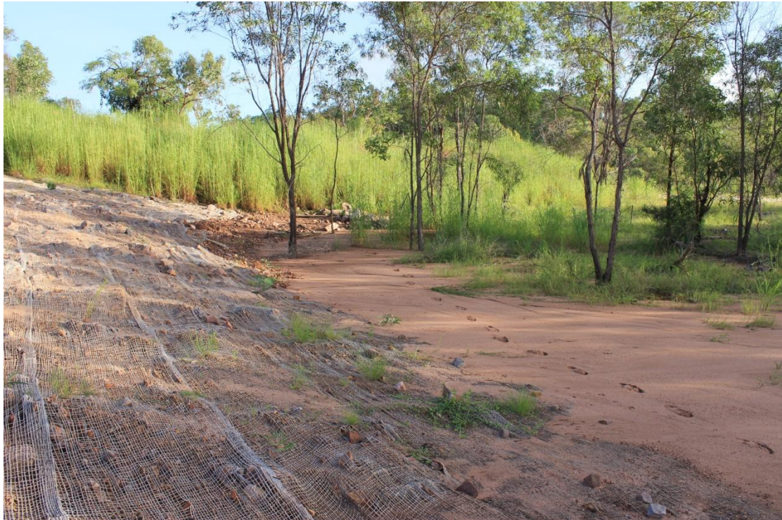
Figure 3 Sediment deposited below the steeper slope in the north western area of the Jabiluka mine site area. Image taken 20-2-2014.
