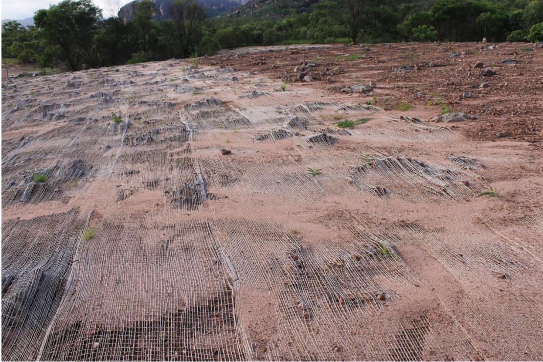
Figure 4 Sand sediment on the steeper slope, some caught in the jute, some being transport downslope across the jute. Image taken 20-2-2014.
