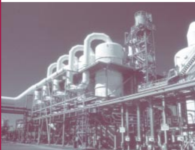
Western Mining Corporation's sulphuric acid plant.
