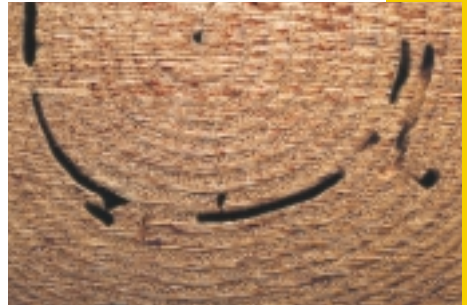
Black carpenter ant damage caused by ants constructing galleries
