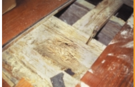
Formosan subterranean termite damage to century old structural timbers
