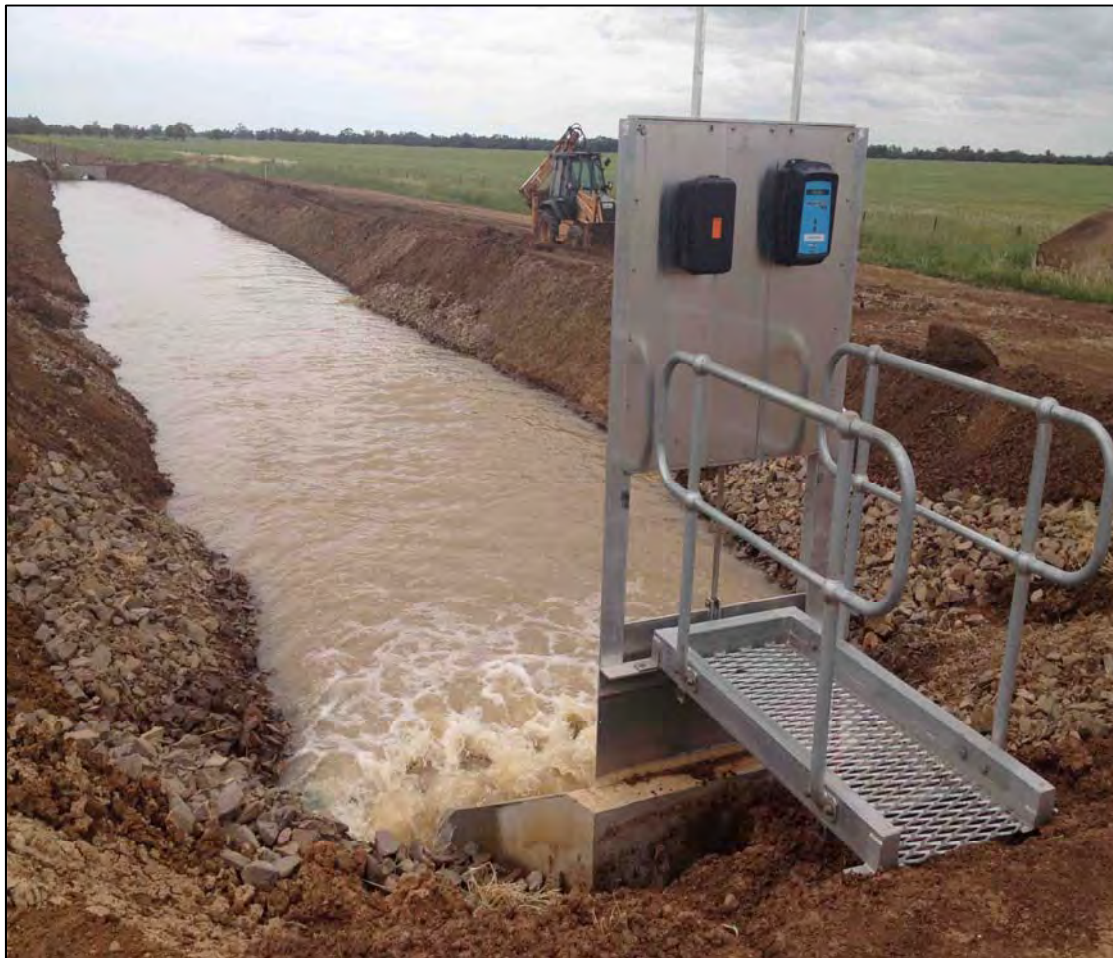
Figure 14: An offtake gate on 'Hatton'. Depending on their location in the channel, offtake gates were fitted with 1200 mm, 900 mm, 750 mm or 600 mm gates, solar-powered electric articulators, MACE flow meters and Observant telemetry systems.
