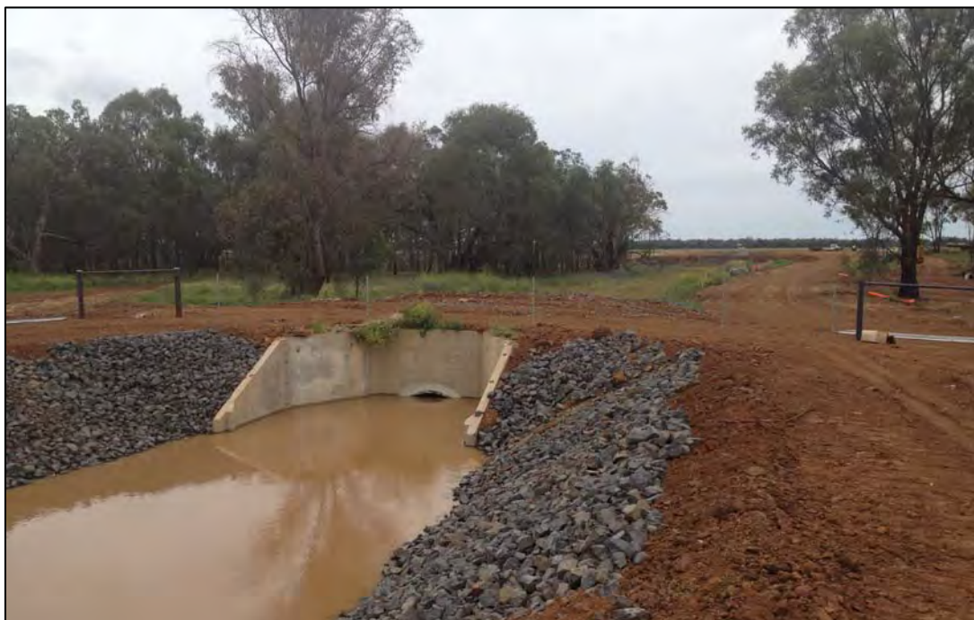
Figure 7: The inlet of Siphon 4, which transfers water beneath the Five Mile Cowal and adjoining floodplain on 'The Cedars'.
