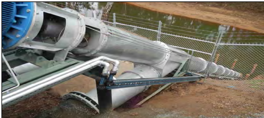
Figure 18: Each of the two new 750 mm multi-stage axial flow pumps installed at Greenhide pump station has a capacity of 130 ML/day.
