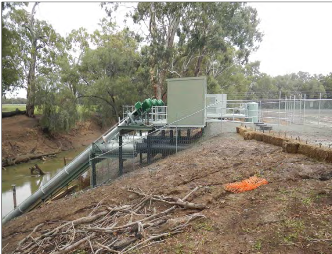
Figure 19: The Gillendoon pump station features three new 630 mm multi-stage axial flow pumps (80 ML/day) with variable frequency drive.
